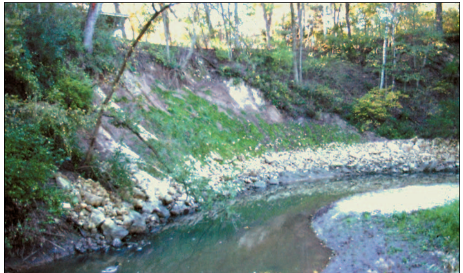
Slope failure endangers a private residence on the Main Channel. Robert Queen, Wisconsin Department of Natural Resources
