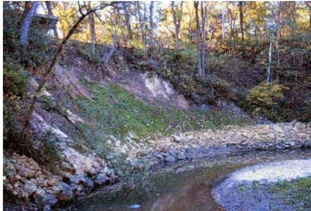
Slope failure endangers a private residence on the Main Channel
