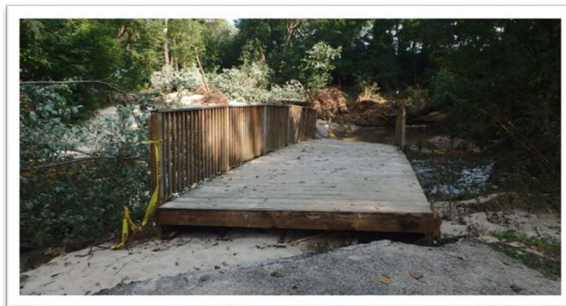
Figure 11: Photo of damaged bridge near Parmenter Street following August 2018 flood viewing downstream (8/25/18).
