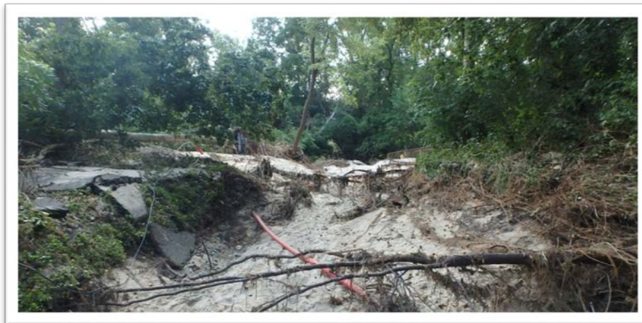
Figure 13: Photo of pedestrian trail damage between Parmenter Street and Park Street following August 2018 flood event (8/25/18).
