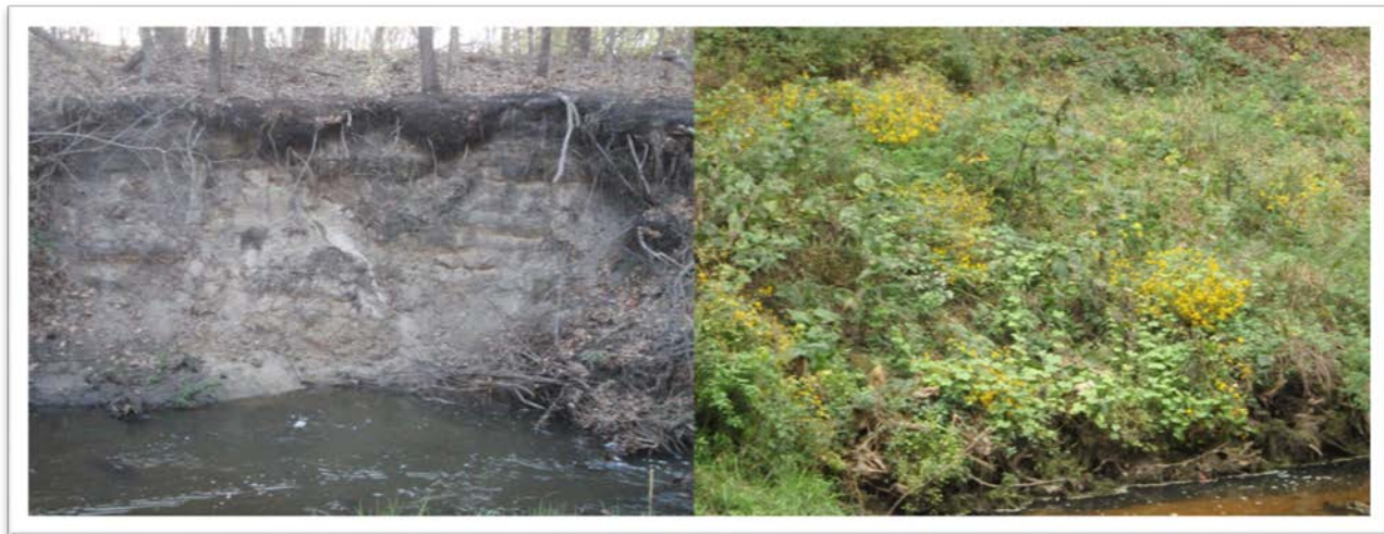
Figure 3: Photo of eroded slope adjacent to Pheasant Branch between Park Street and Parmenter Street in 2010 (left) and same slope after construction taken in 2014 (right).
