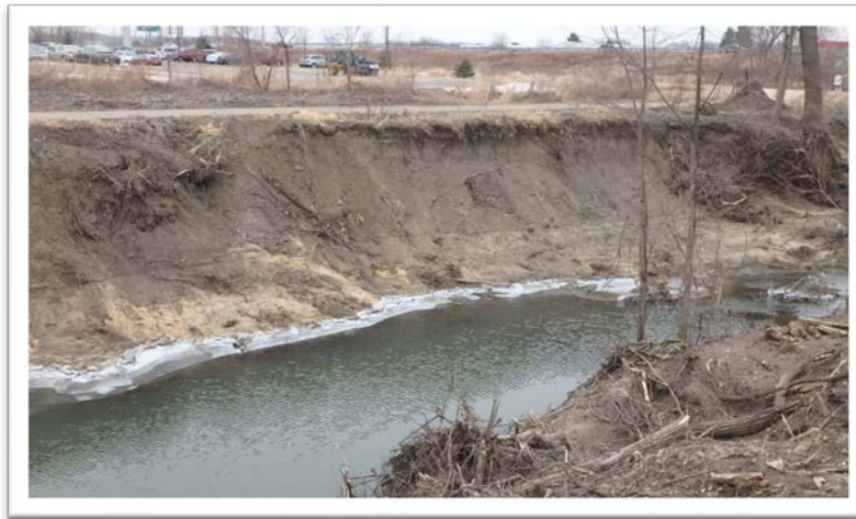
Figure 10: Extreme streambank erosion as a result of August 2018 flood event near Deming Way viewing downstream (1/15/19).
