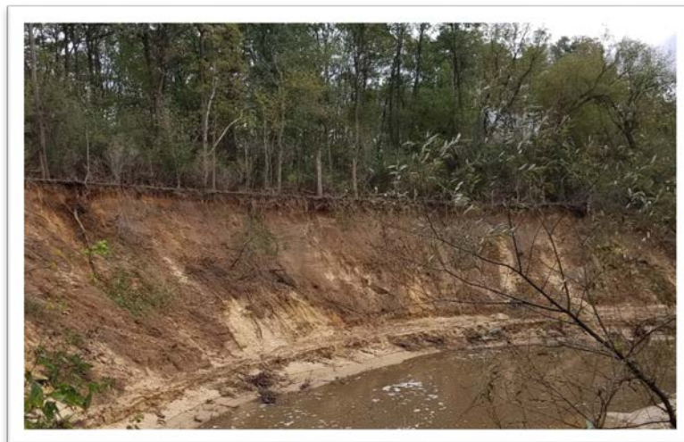
Figure 15: Photo of extreme streambank erosion directly downstream of Park Street as a result of August 2018 flood event (10/11/18).
