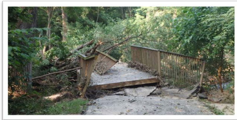
Figure 14: Photo of damaged pedestrian bridge between Park Street and Century Avenue following August 2018 flood event (8/25/18).
