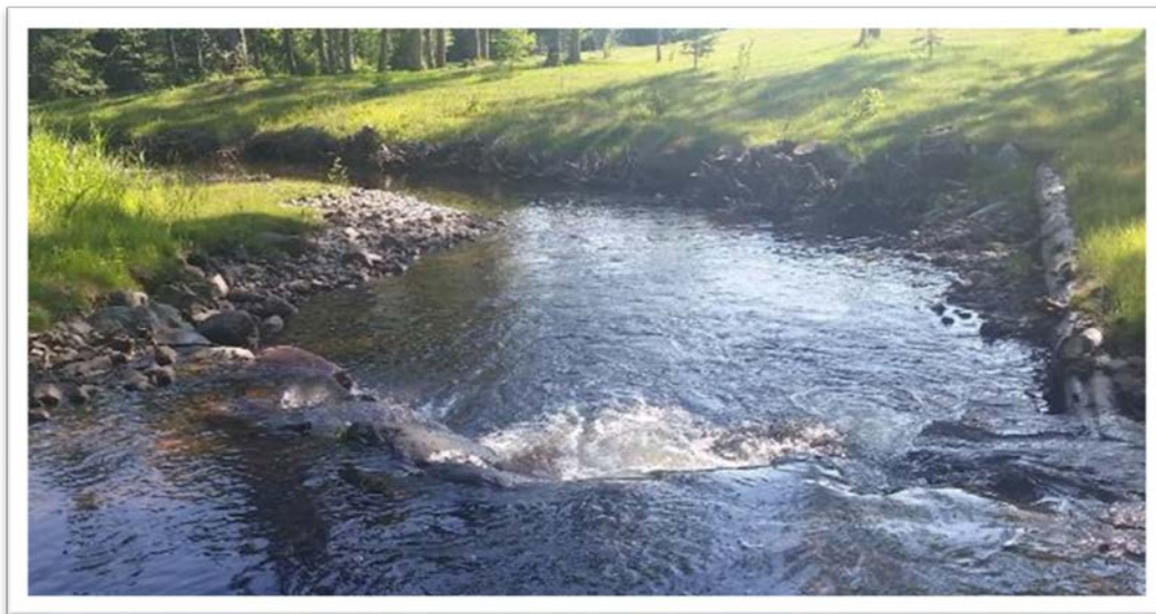
Figure 64: Example of rootwad log vane J-hook combination installed by Cardno on the Knife River in 2016 near Two Harbors, MN
