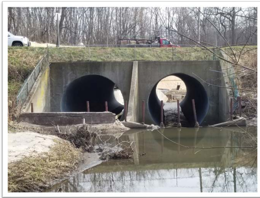
Figure 67: Photo of Park Street fish barrier
