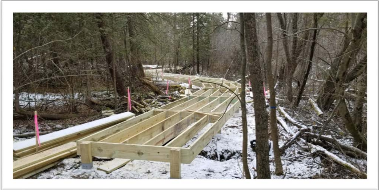
Figure 48: Example Bridge Pan style substructure. Pans are located at each of the posts on the snow
