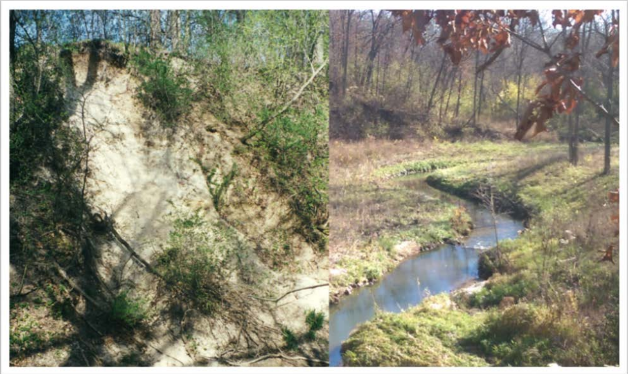
Figure 4: Photo of collapsing streambank adjacent to Pheasant Branch near site of Kromrey Middle School addition 2013 (left) and same section of stream after construction taken in 2016 (right).
