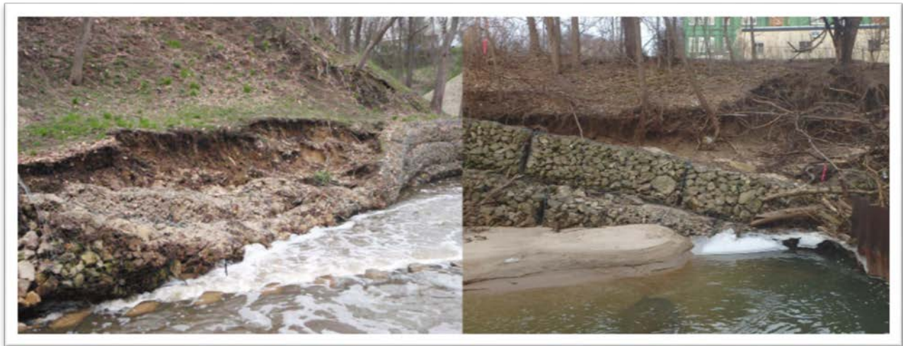
Figure 66: Photo of failed gabion baskets between Park Street and Century Ave taken in 2008 (left) and directly downstream of Century Ave taken in 2018 (right).
