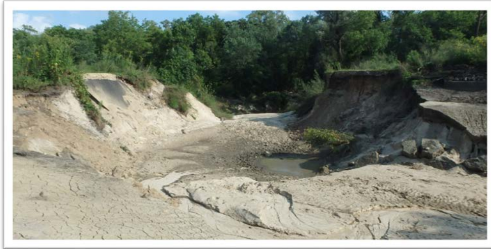
Figure 12: Photo of Donna Dr. sedimentation pond failure following August 2018 flood event (8/25/18).
